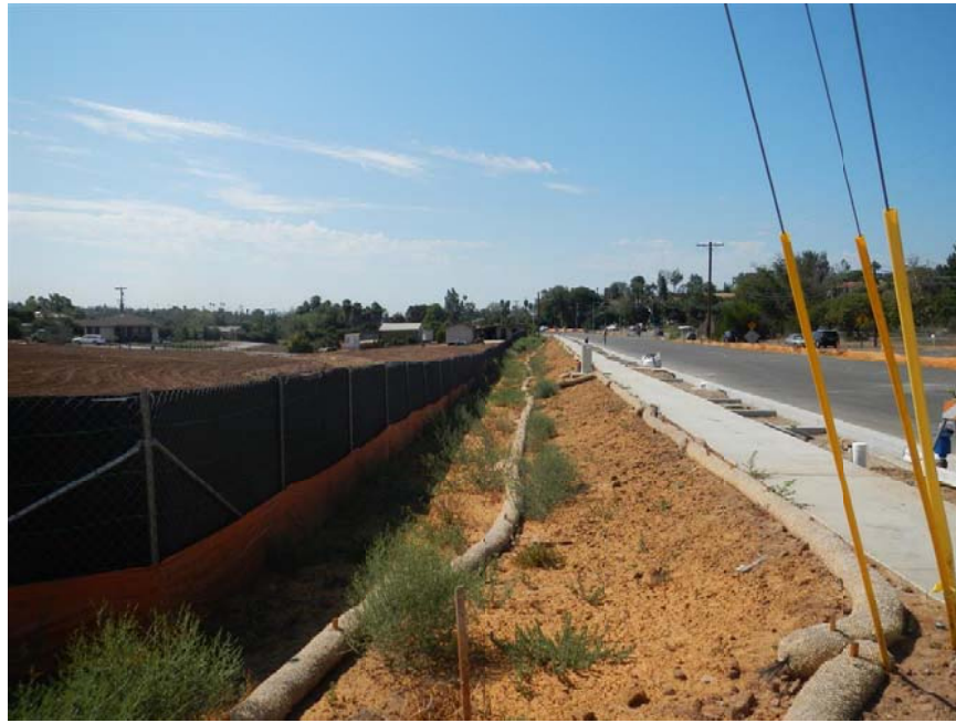
Photo #3: View to south from northwest corner of site; subject property on left and Bear Valley Parkway is on right
