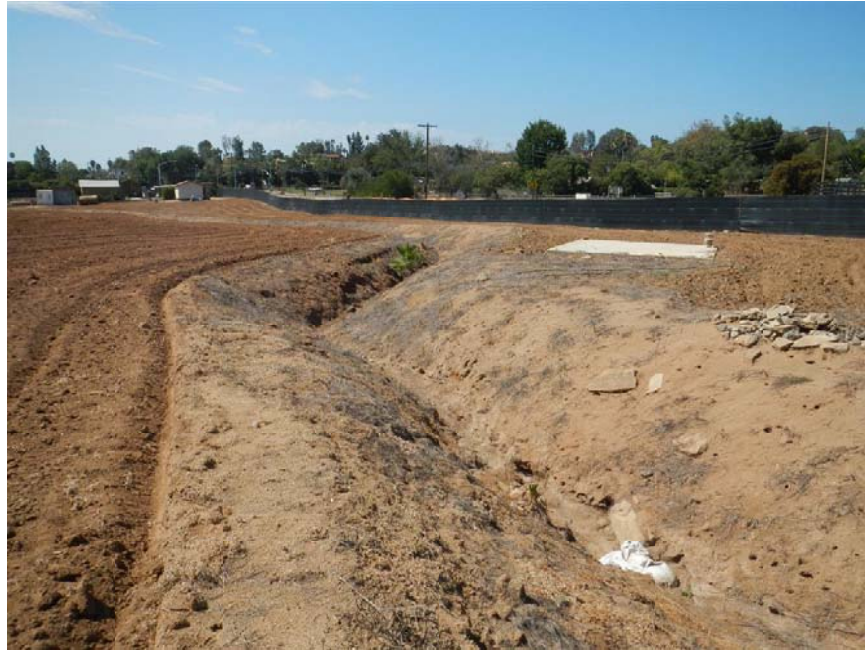
Photo #7: View of west drainage channel from north to south. Concrete slab and minor concrete debris on right.
