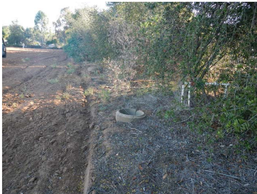
Photo #12: Water services and former agriculture appurtenance on east margin of property.
