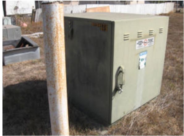
Photo #38 One of two pad-mounted transformers located on the southwest portion of the site (owned and maintained by SDG&E).
