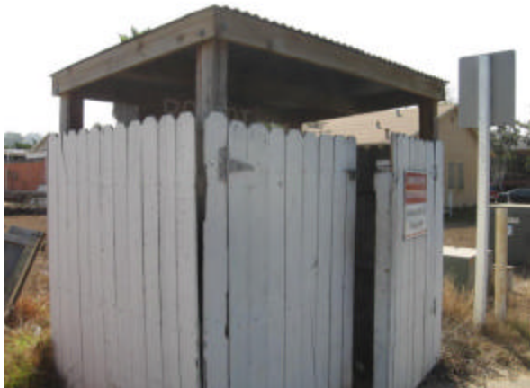
Photo #39 Small municipal trash shed located on the southwest portion of the site along Sierra Avenue.
