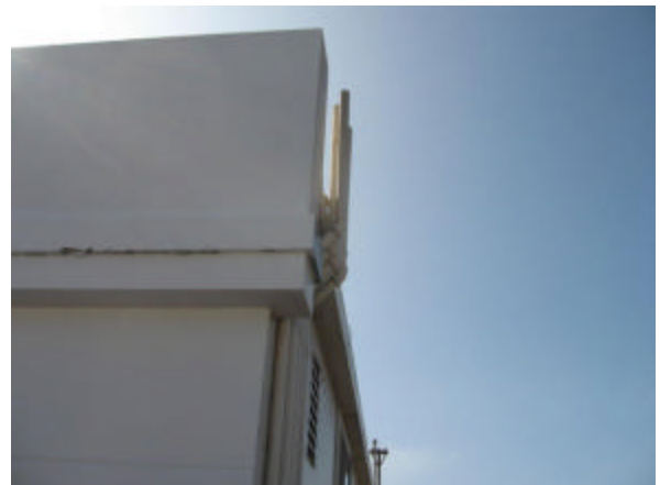
Photo #24 Remaining vent pipes of former gas station USTs, northwest corner of building at 343 South Highway 101.
