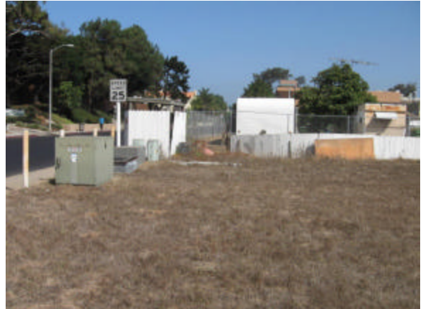
Photo #8 Yard area behind vacated house at 128 Dahlia Drive. Pictured at left are two pad-mounted transformers (owned and maintained by SDG&E).
