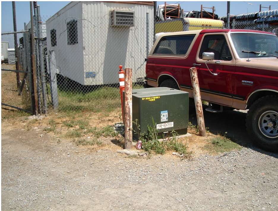
Photograph #21 View of typical pad-mounted transformer at Site (one of four) located in northwest portion of Site on north side of central road.
