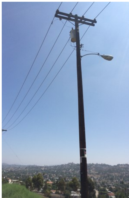
8. Transformer on south side of property.
